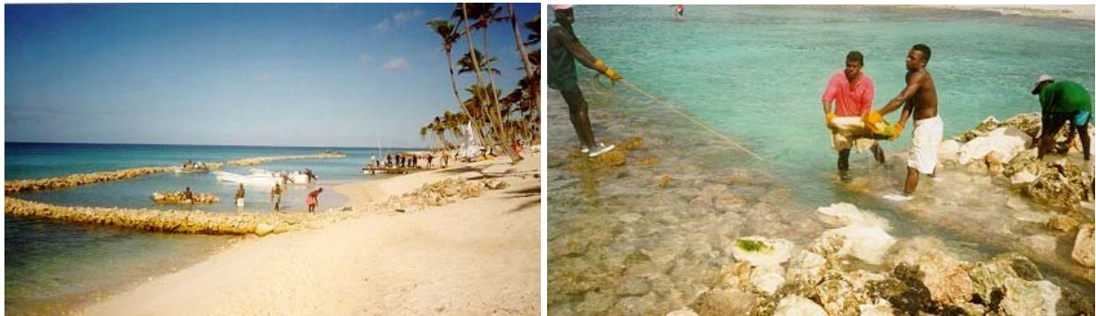
Figure 6. Placement of Small Rocks on top of Submerged Reef Ball™ Breakwater. Photograph taken in February 1999 during construction.
