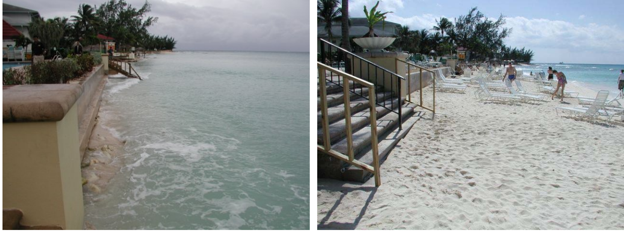
Figure 6. Before and After Breakwater Installation Photographs – View South October 2002 (left) and February 2003 (right)
